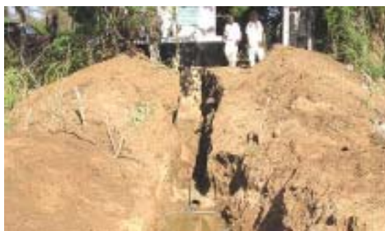
Infiltration pipe connecting to the intake.
