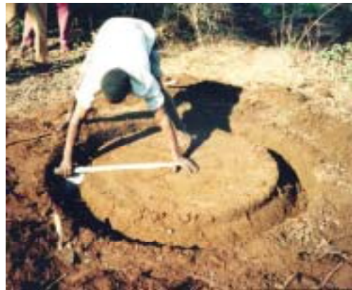
A groove being cut for a foundation ring with the tool seen above. The groove will be filled with reinforced concrete.
