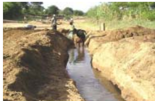
A flooded trench for infiltration pipes.
