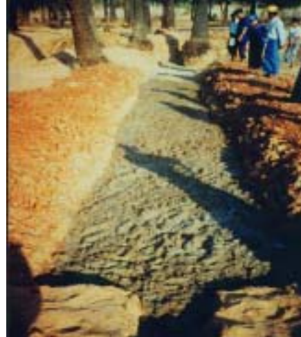
The excavation is being filled with compacted moist clayey soil by a community in Myanmar (Burma)
