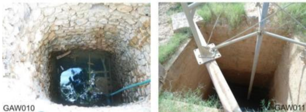
Figure 5.20 a,b Dug wells in Nugaal region - different types and intake structures
