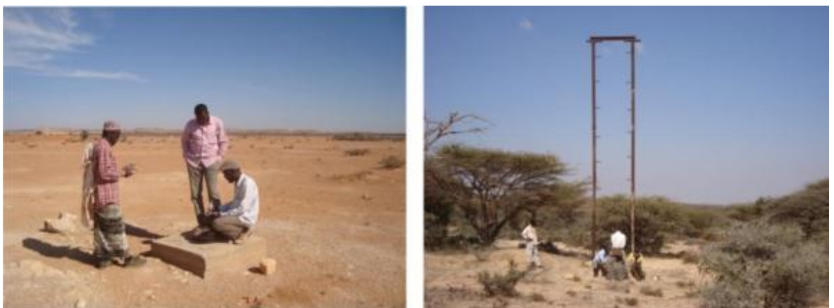
Figure 5.18 a,b Drilled wells: QAB001 (left) and QAB006 (right) in Bari Region
