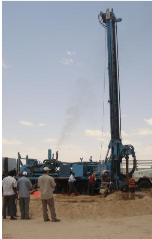
Figure 5.67 Drilling of a new well in Xumba Weyne for Hargeysa water supply. The adequate groundwater protection measures must be taken in consideration along with building of a new infrastructure (pump rooms, pipes, chlorinators, etc.)
