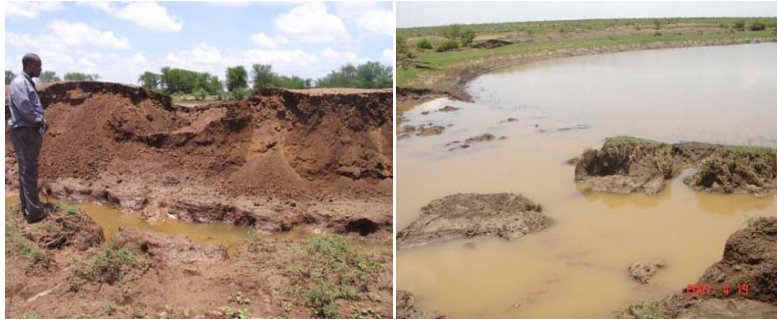
Figure 5.3: Impacts of Allaybaday flash floods: a photo of a broken sand dam in the area due to a recent flash flood 10
