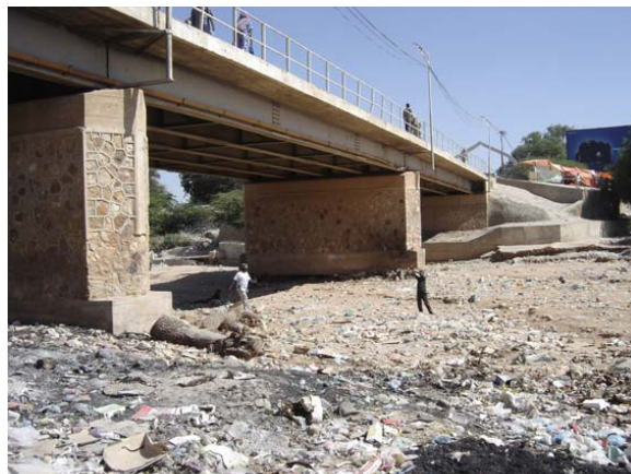
Figure 5.2: Bridge in Hargeysa on the Marodi Jeex Wadis that was washed away during the flash flood event of May 2005
