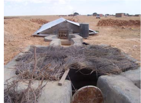
New-model berked with iron roof, constructed by COOPI in Sibaayo
